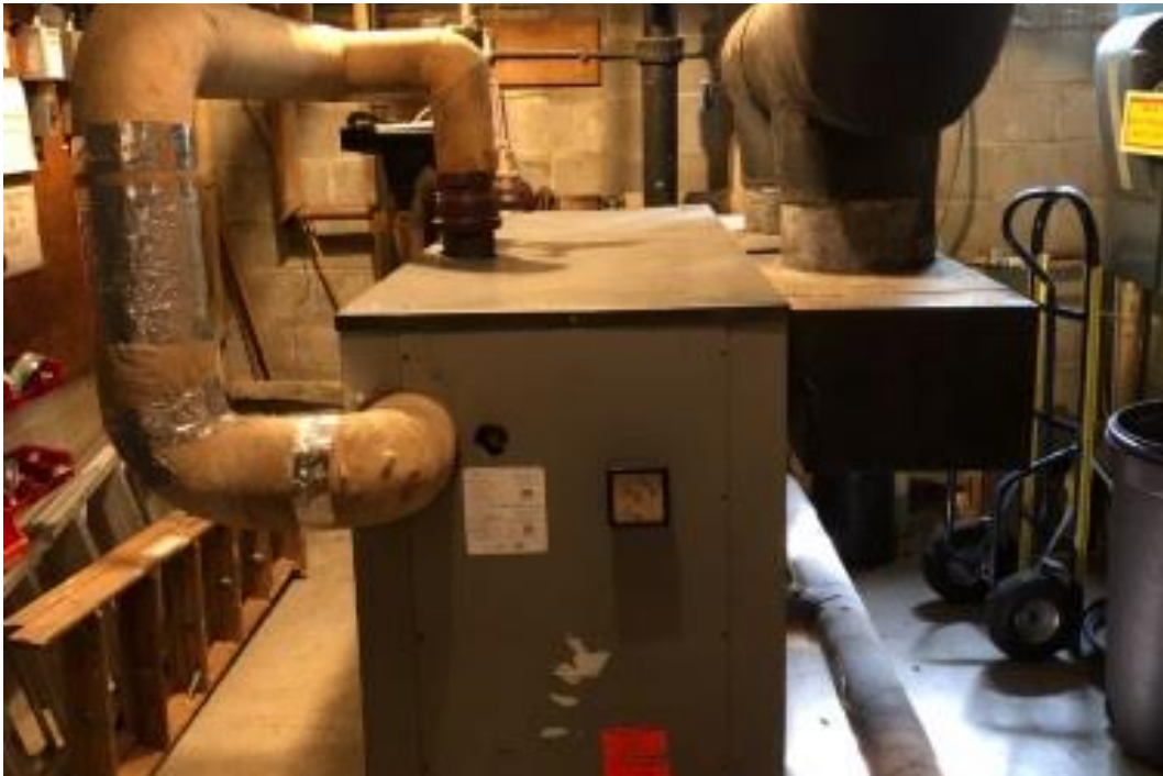
Old Boiler at UUFM
