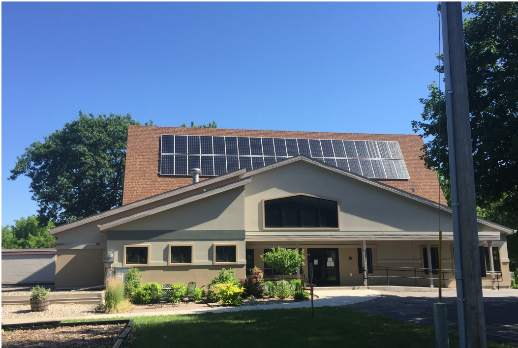
UUFM Building with Solar Array
