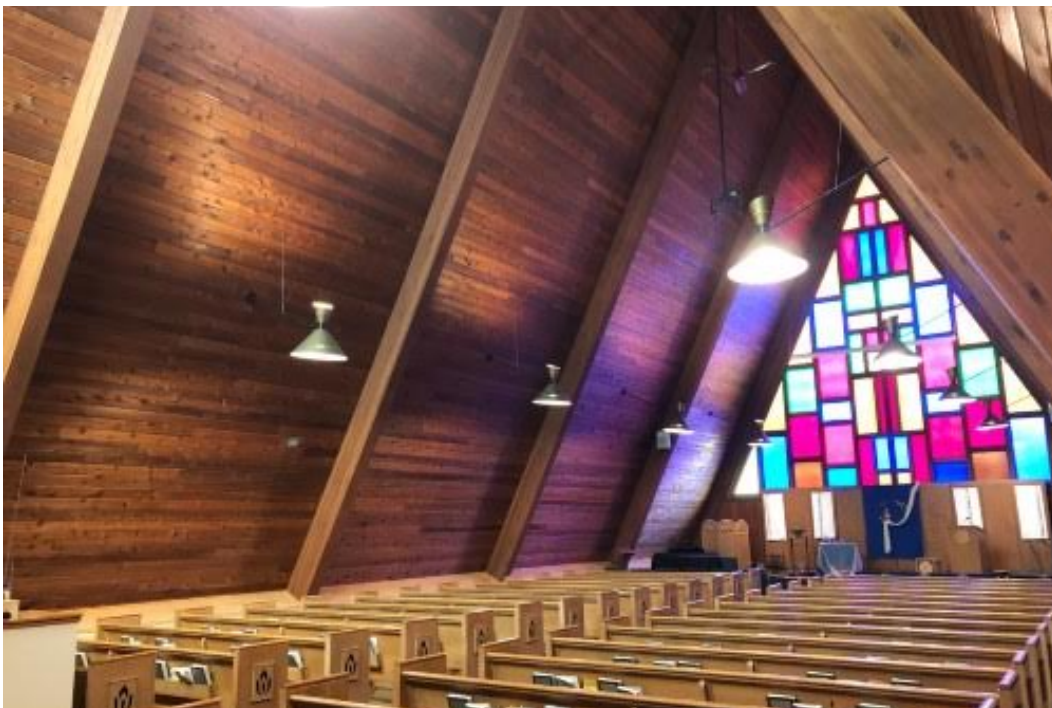
LED Lighting in Sanctuary UUFM
